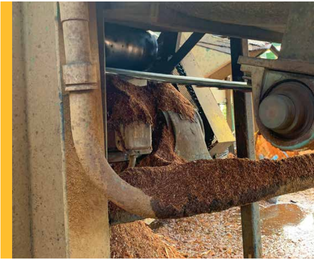
Replacing the entire competitive gearmotor assembly was expensive and labor-intensive, requiring two skilled millwrights 4 hours to complete.
