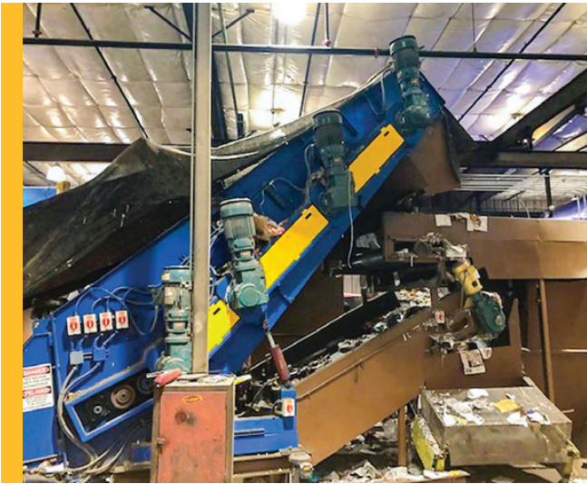
The baler incline conveyor with Quantis gearmotors ensures material continuously flows to the next recycling phase.
