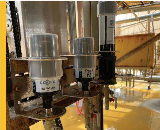
Since installing OPTIFY Intelli-Lube, the plant has seen an immediate positive impact to operations with no pump failures in over 1 year.
