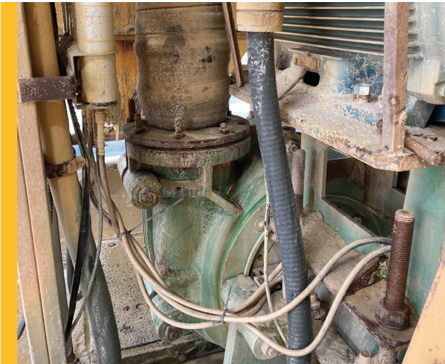
Contamination ingress due to environmental conditions led to slurry pump failures every 2 weeks.
